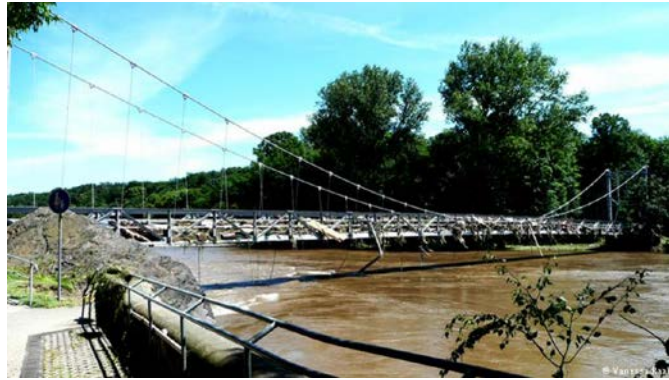
Figure 35 Suspension bridge covered in debris on June 6th 2013 (DW, 2013)
